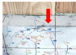
Fig.8 Damage of beam
