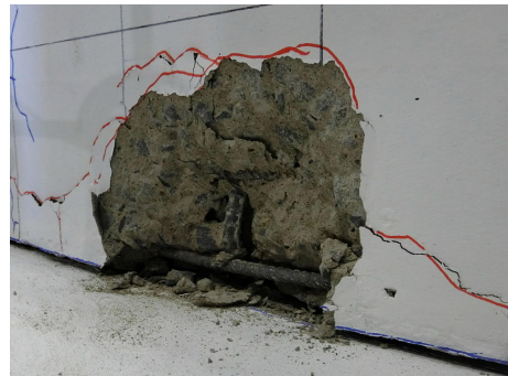
写真-1 補強軸方向鉄筋の座屈 (No.1)
